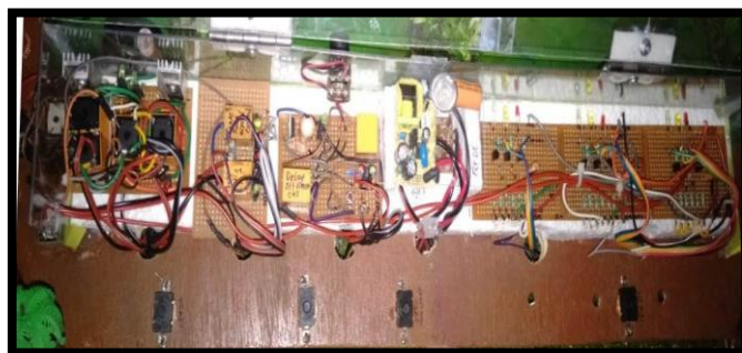
Figure 8: Circuit Control Box
